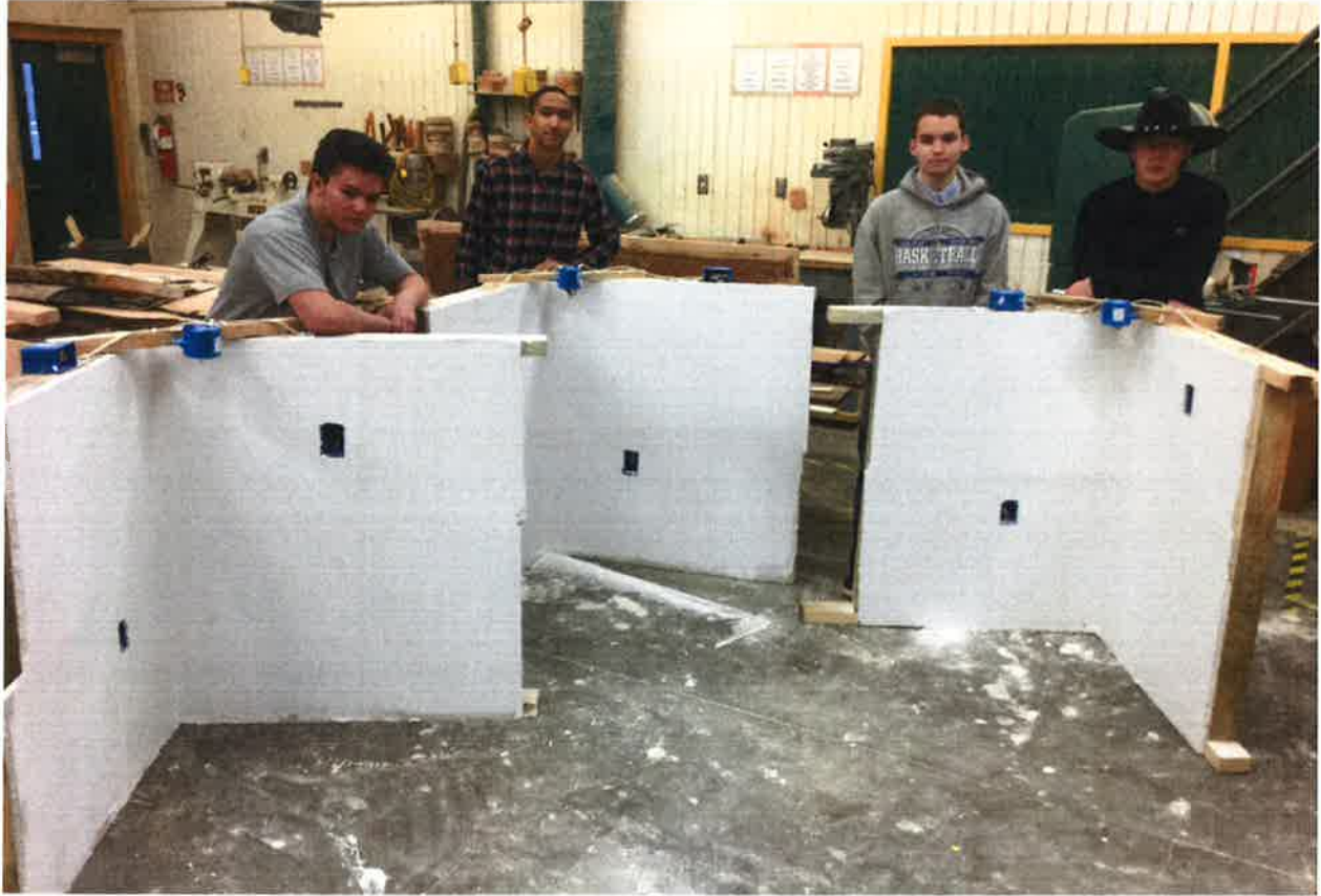
Mr. Schott's Career Explorations Class completed their project starting with framing, wiring, drywall and painting.
